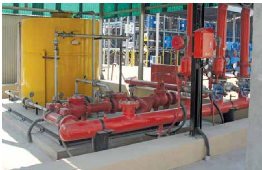
Automatic foam based sprinkler system
