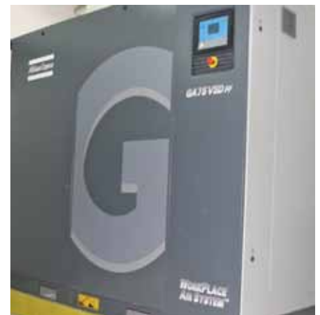
A view of the inverter driven compressors installed
